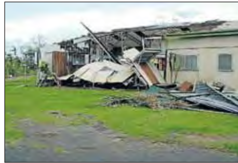
Cyclone Yasi caused widespread damage to infrastructure, but the recovery behind the scenes is lengthy as well.
